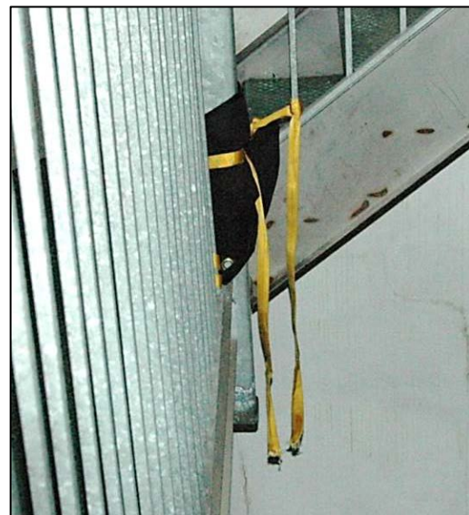
Figure 9- Upper anchor point following failure of nylon webbing.
